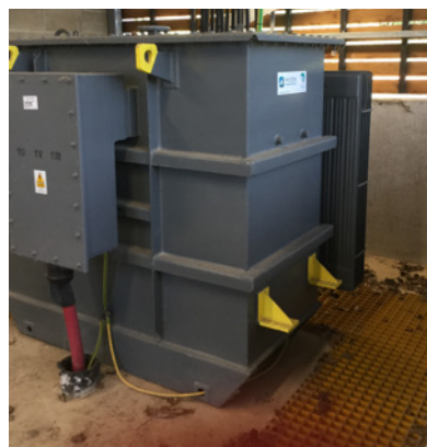
1000kVA Wilson e2 transformers in the Barton & Hickling Residences Substation
