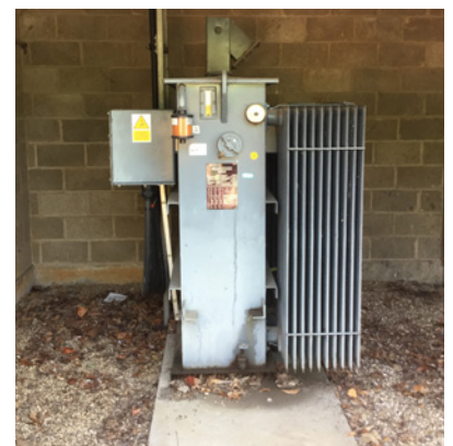
1000kVA South Wales Switchgear Transformer from 1960
